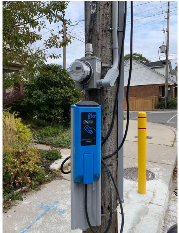
On-street EV charging station on a hydro pole, Toronto
